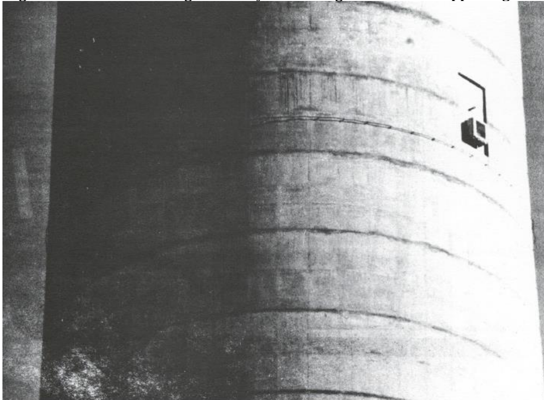
Figure 14-2. High-intensity obstacle lights installed on a chimney
